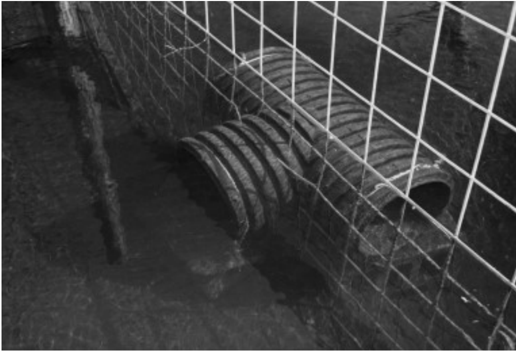
Photo 4. A 30 cm polyethylene T-joint in the front of this Beaver Deceiver™ keeps beavers and large turtles out of traffic by allowing them to travel through the fence and therefore the road culvert. The 90° angle prohibits beavers from transferring woody damming material inside. Photograph: Skip Lisle.
